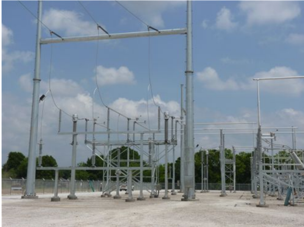
Figure 6: Termination Towers with H-Frames
